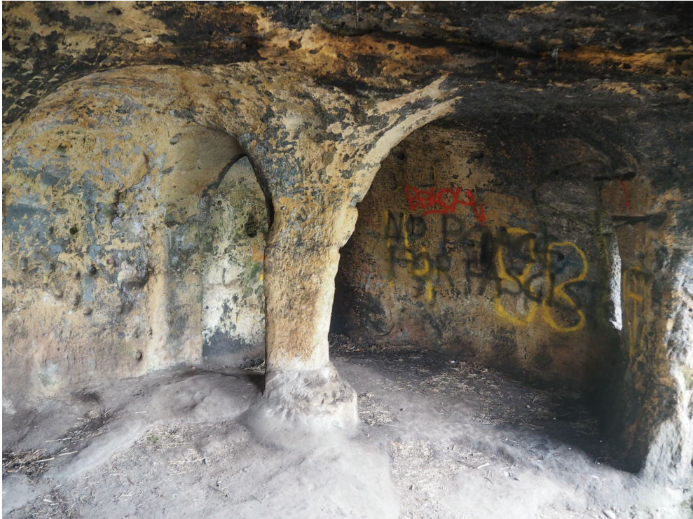
Figure 5. Former dividing wall between rooms A1 and A2. The door (complete with bolt hole and channel for frame) is on the left side, the opening on the right is the result of demolition.
